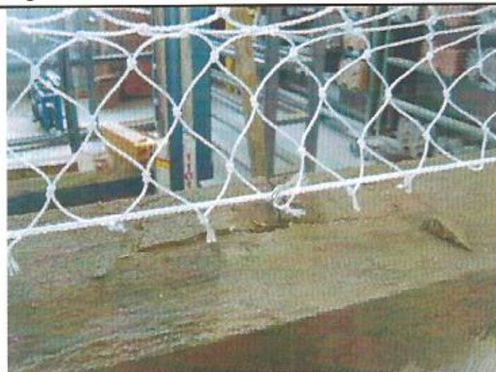
Fig. 2 – Details of hook and anchor slippage at the central bottom part of frame
